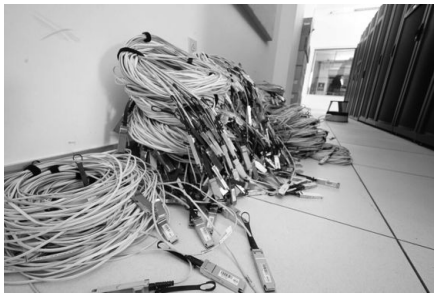
Stacks of InfiniBand QSFP Fiber/Active Optical Cables after being tested.
